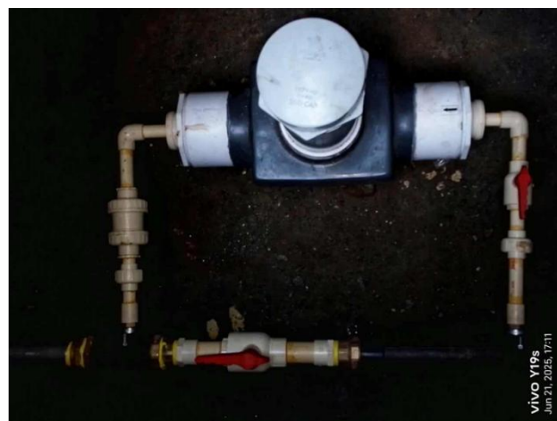
Inline Chlorination unit in DWSS of Ghoyalneta
